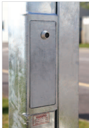
All columns have flush fitting doors
